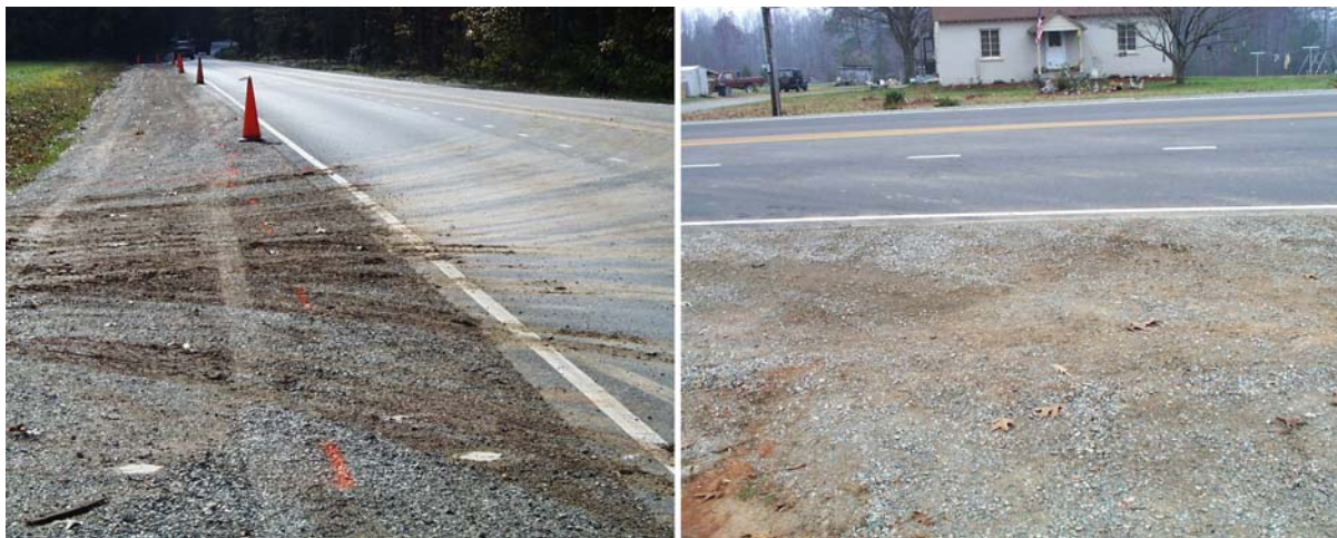
Figure 7. Conditions at Field Entrance on Two Dates. Left, October 26; right, November 22.
