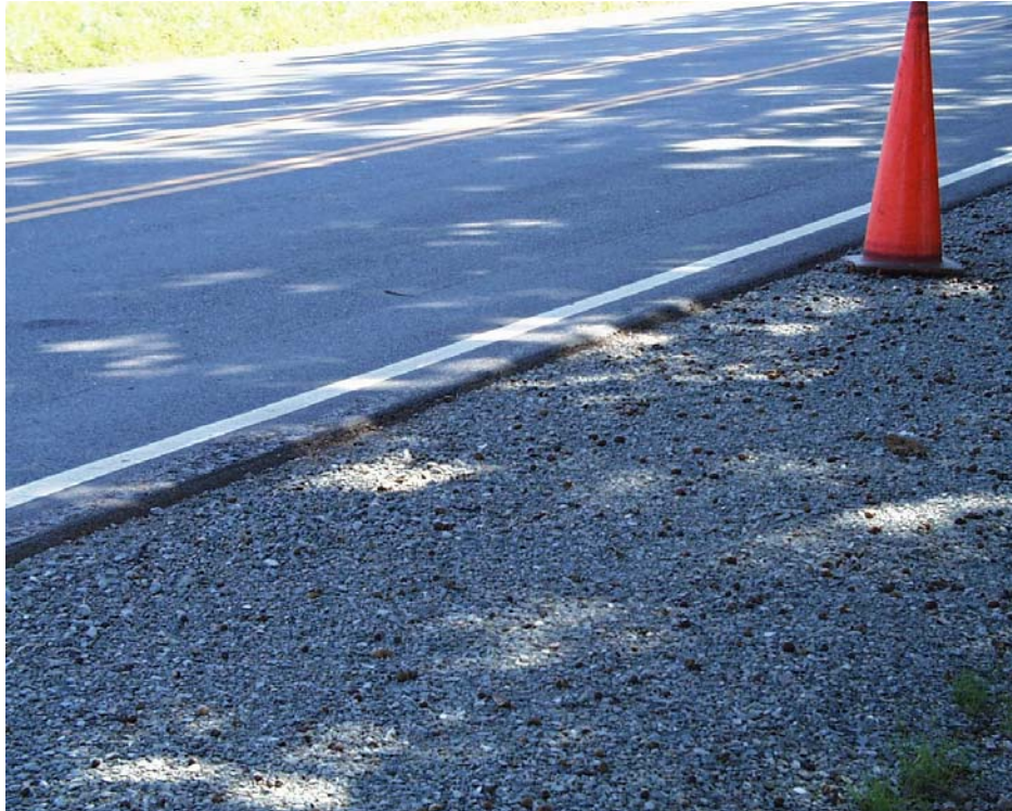
Figure 4. Low Shoulders Along Control Section, 10/6/2004
