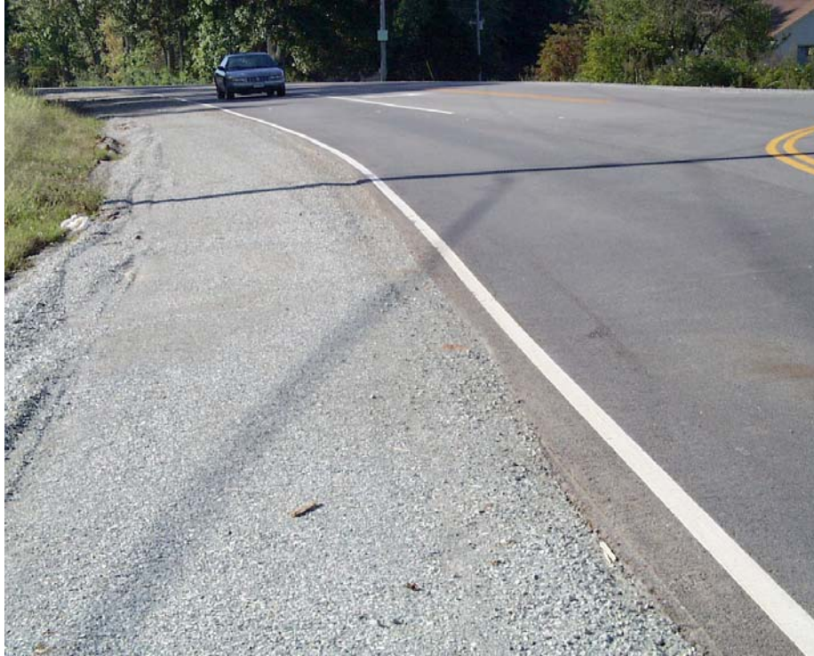
Figure 3. Low Shoulders along Soiltac Test Section, 9/21/2004
